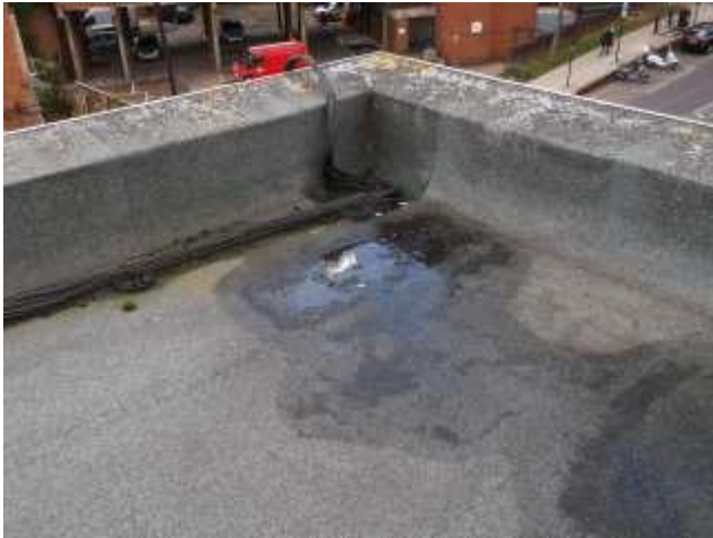
Above: Mineral felt flat roof in reasonable condition for its age requiring some repairs and cleaning off and resealing of outlets.
