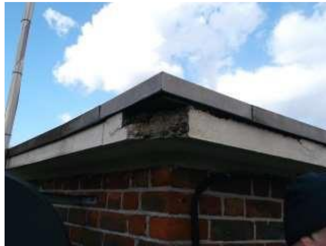
Above: Concrete soffit/fascia to tank room roof requiring repairs
